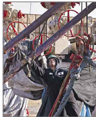
Leaks of tons of methane from oil and gas facilities are contributing to climate change.
